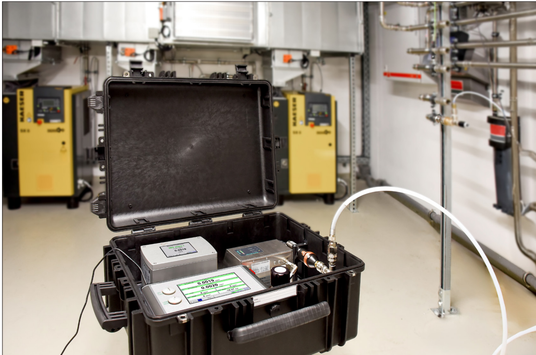
Application: Measurement in the compressor room - OIL CHECK 500- DS 500 - PC 400
